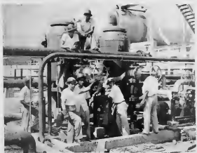
PUMPS REPLACED: There's no substitute for safety, so Lago has replaced three pumps which were considered a safety hazard. Recently these two new pumps, with explosion-proof motors and a 36,000 gallon-per-hour capacity, were installed in the Low Octane Stabilizer and Splitter plant. Both the vertical-type pumps and the motors are located inside a weather-proof housing in contrast to the previous installation which had the motors and the pumps separated.
